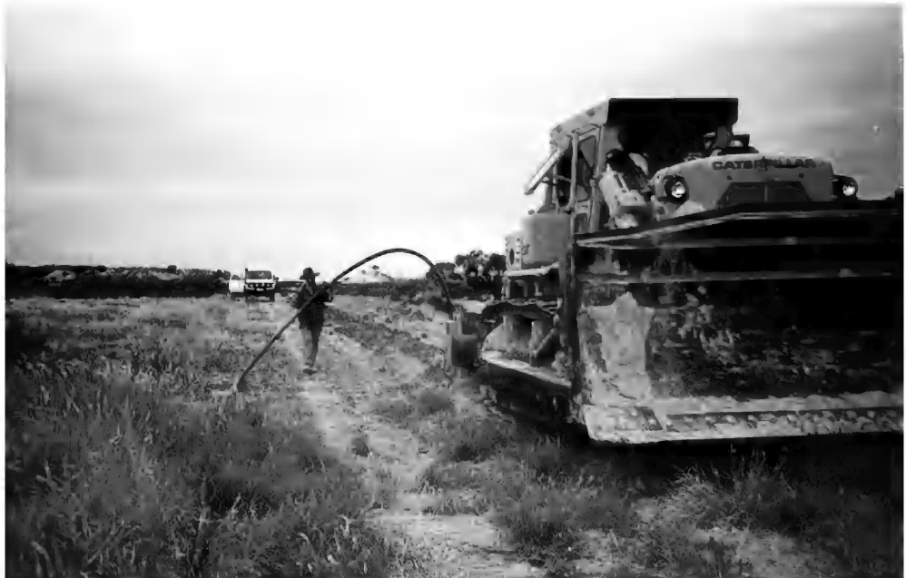
Figure 8. Replacement of bore drains with polypipe to create closed water systems (Source: DNRME).
